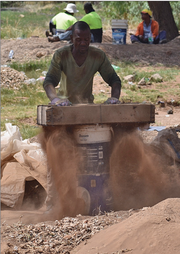
Figure 4. Dust exposure from sieving, lack of respiratory PPE (2018) (Square Hill Park) Photograph: André Rose
