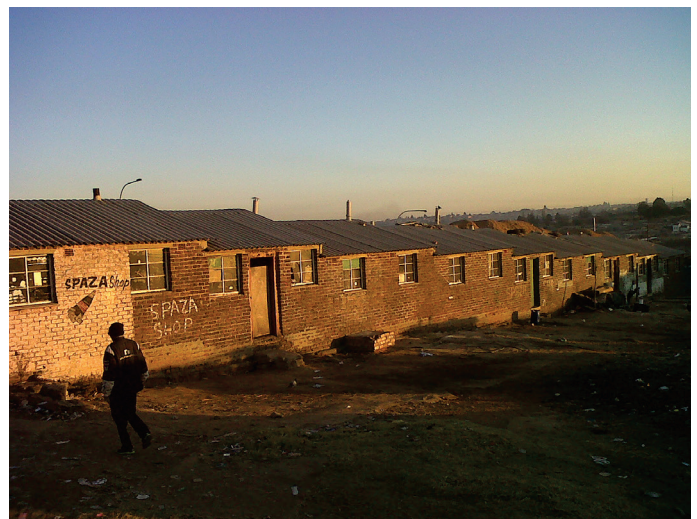
Asbestos cement roofs in Soweto Photo: D Africa
